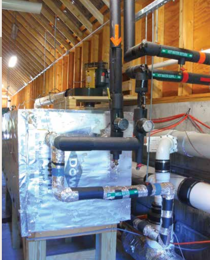
Mechanical room with view of heat exchange unit. Photo courtesy of John Aber
